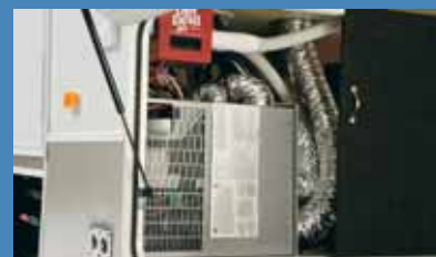
A sliding door provides handy access to the furnace, central vacuum and other mechanic items.
